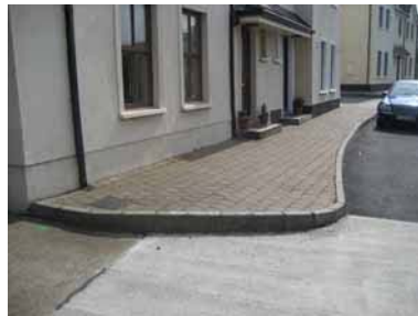
(g). High curb, not dished out.
